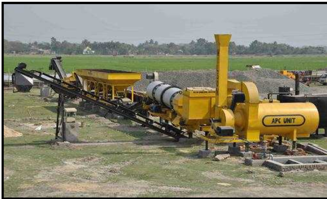
Figure 4: Existing Hot Mix Plant (HMP)
