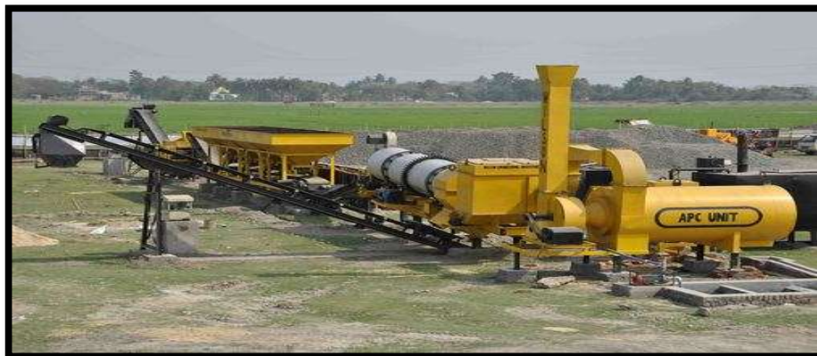
Figure 4: Existing Hot Mix Plant (Drum Mix)
