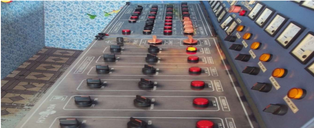
Fig. 4: Control panel of Hot mix plant
