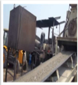
Aggregate feeding to the Drum Mixer through Conveyor Belt
