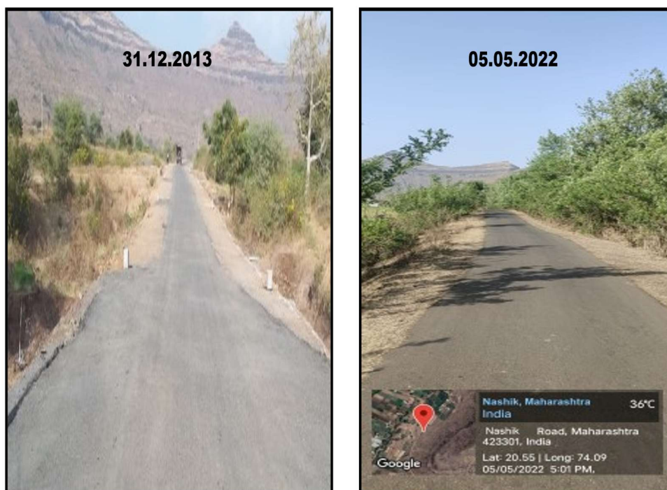
Proven 8 Years Surface Life of Tailor-made Coldmix Road executed in 2014 at Pandhripada, Nashik-Maharashtra, India as on May, 2022
